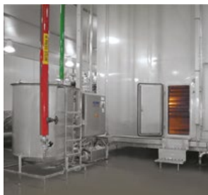
Full recirculating cleaning system
